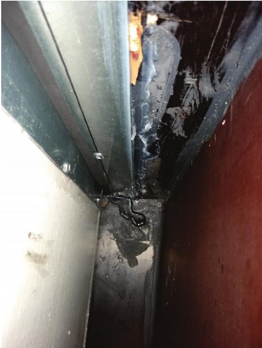
Photo B. 6.9 Leakage of 500 mm test, water at the outside
