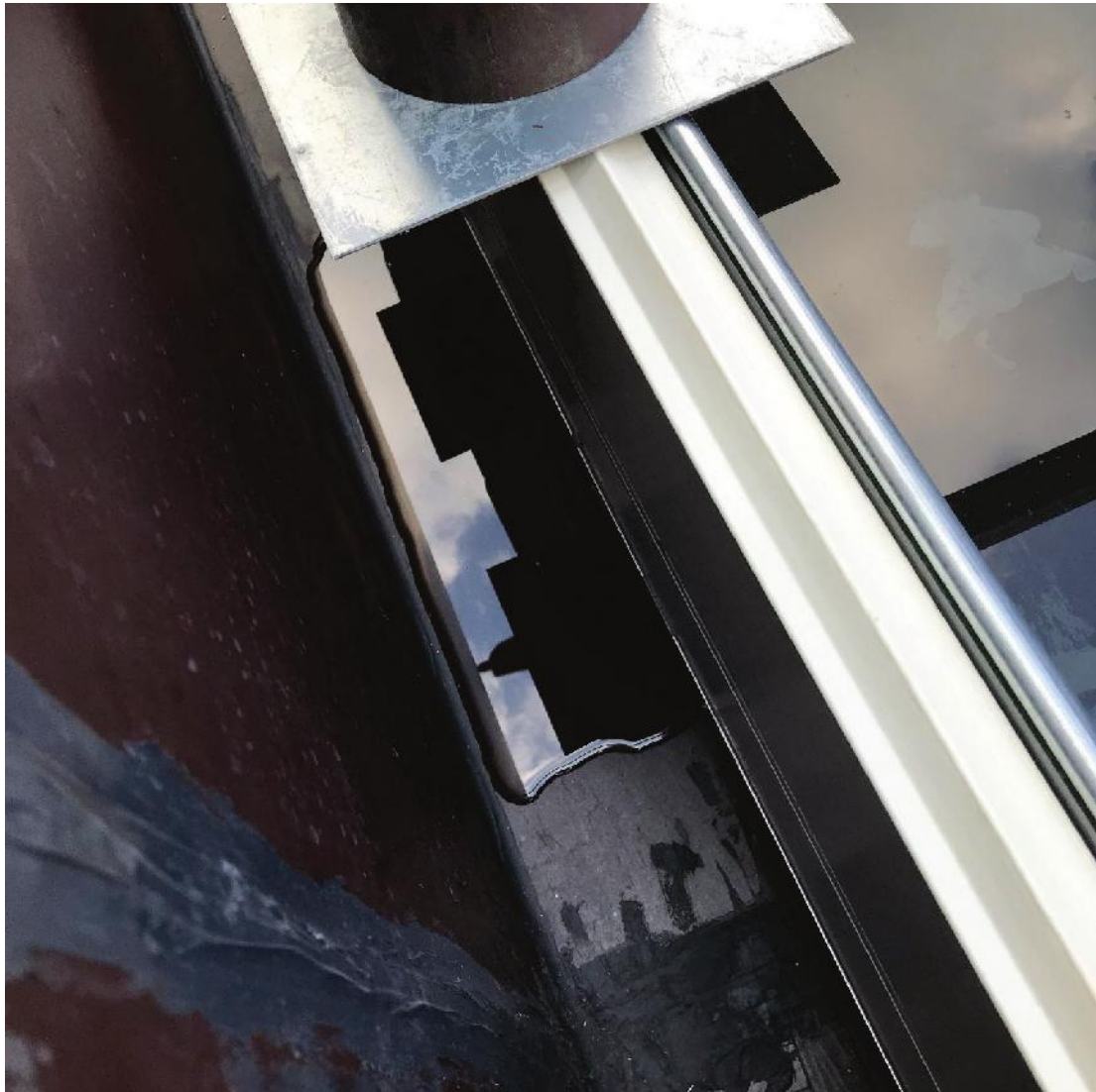
Photo B. 3.9 Leakage of 300 mm test, water at the inside
