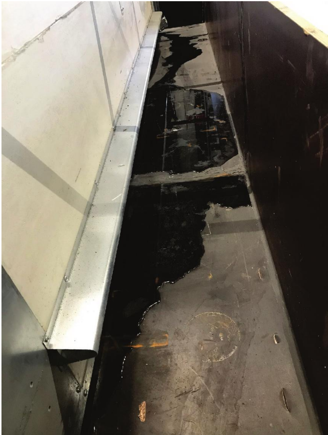
Photo B. 9.9 Leakage of 300 mm test, water at the inside
